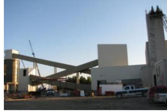
Transfer Towers & Conveyors
