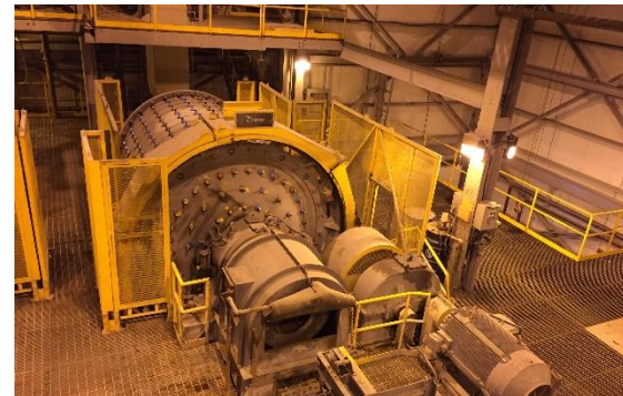
Existing Ball Mill
